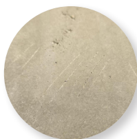
Carbonated concrete core with soft chalky surface.
